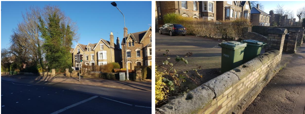
Above Left: 101-105 Lincoln Road. All of these properties had railings removed. Right: 103 Lincoln Road. The holes left after the railings were pulled out can still be clearly seen.
