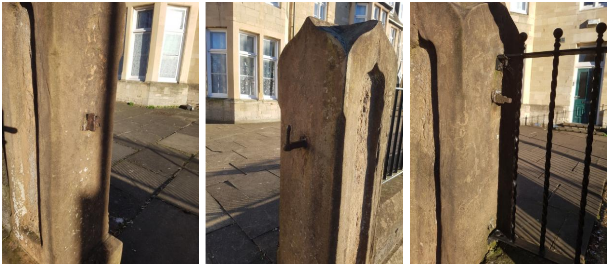
Above: 71-73 Lincoln Road. The first image shows a bracket against which a small gate would have rested when closed. The second image shows the hinge pin on the opposite side where the iron gate would have hung. The third image shows where the old railings were cut off, behind which, modern railings have now been installed. This wall stretches quite a long way in front of a long row of buildings.
